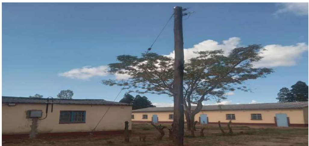
Mwaruta Primary School Electrified
