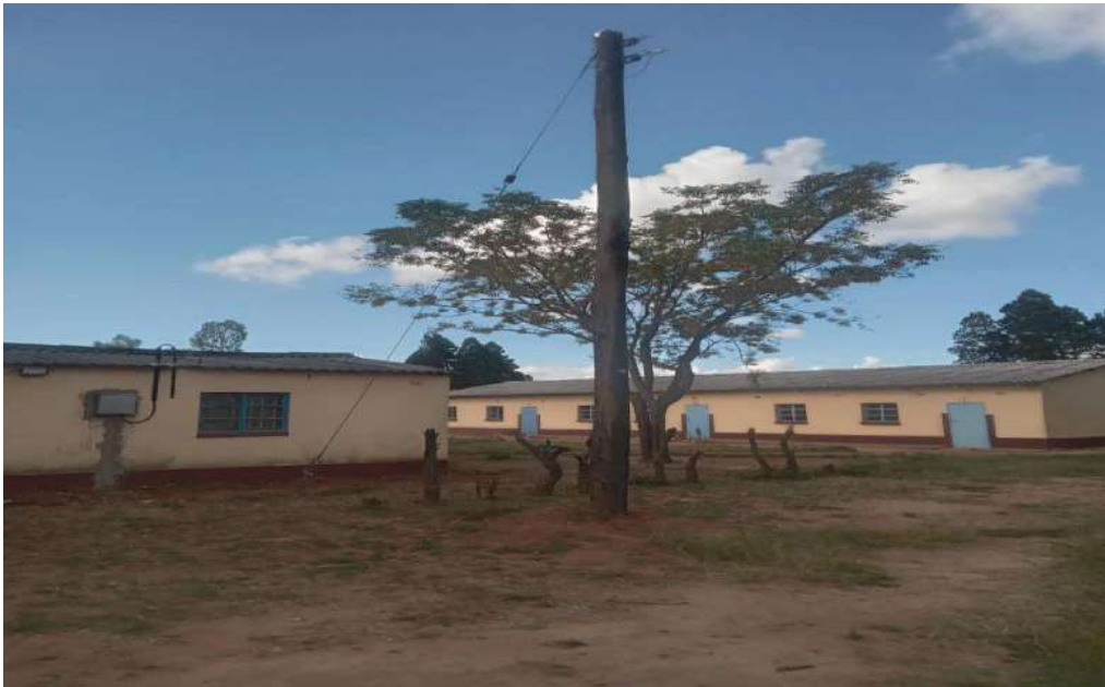
Mwaruta Primary School Electrified
