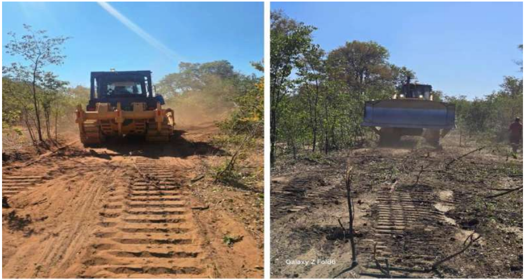
Bush clearing on detour construction (Insiza and Cross Jotsholo) for the Rehabilitation of Bulawayo Victoria Falls Road
