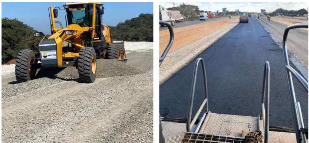
Processing of G1 (Base Material)-16kms from Masvingo Urban towards Beitbridge and Surfacing from Chinzou Traffic Circle to Willowvale Junction (North Bound lanes).
